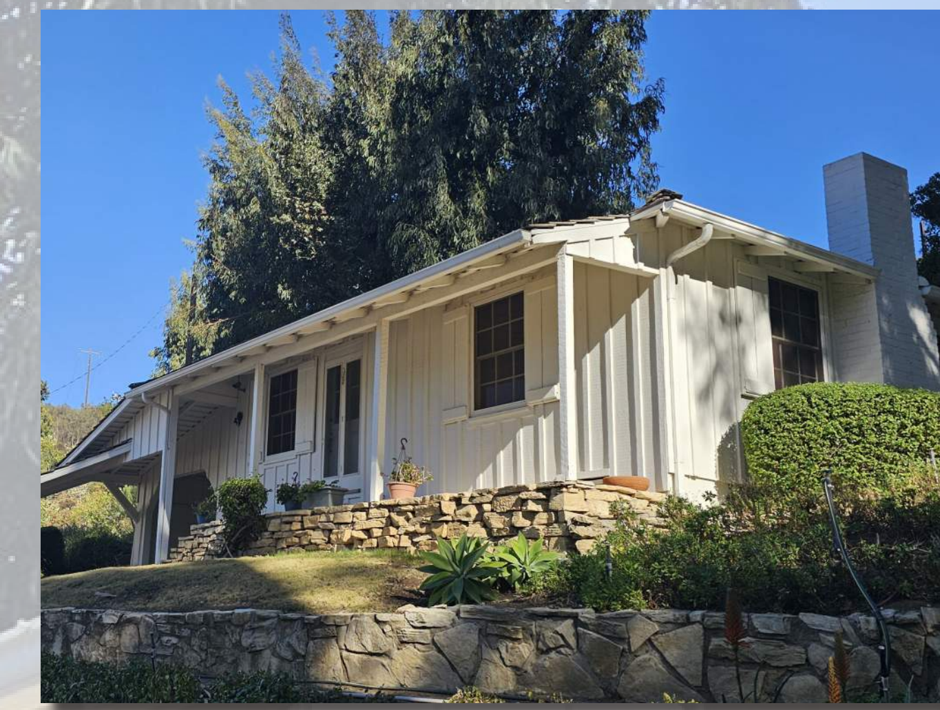
REPAIR/RESTORE EXTERIOR COMPONENTS (ROOF, SIDING) (2026 Est. Cost $41,800)
