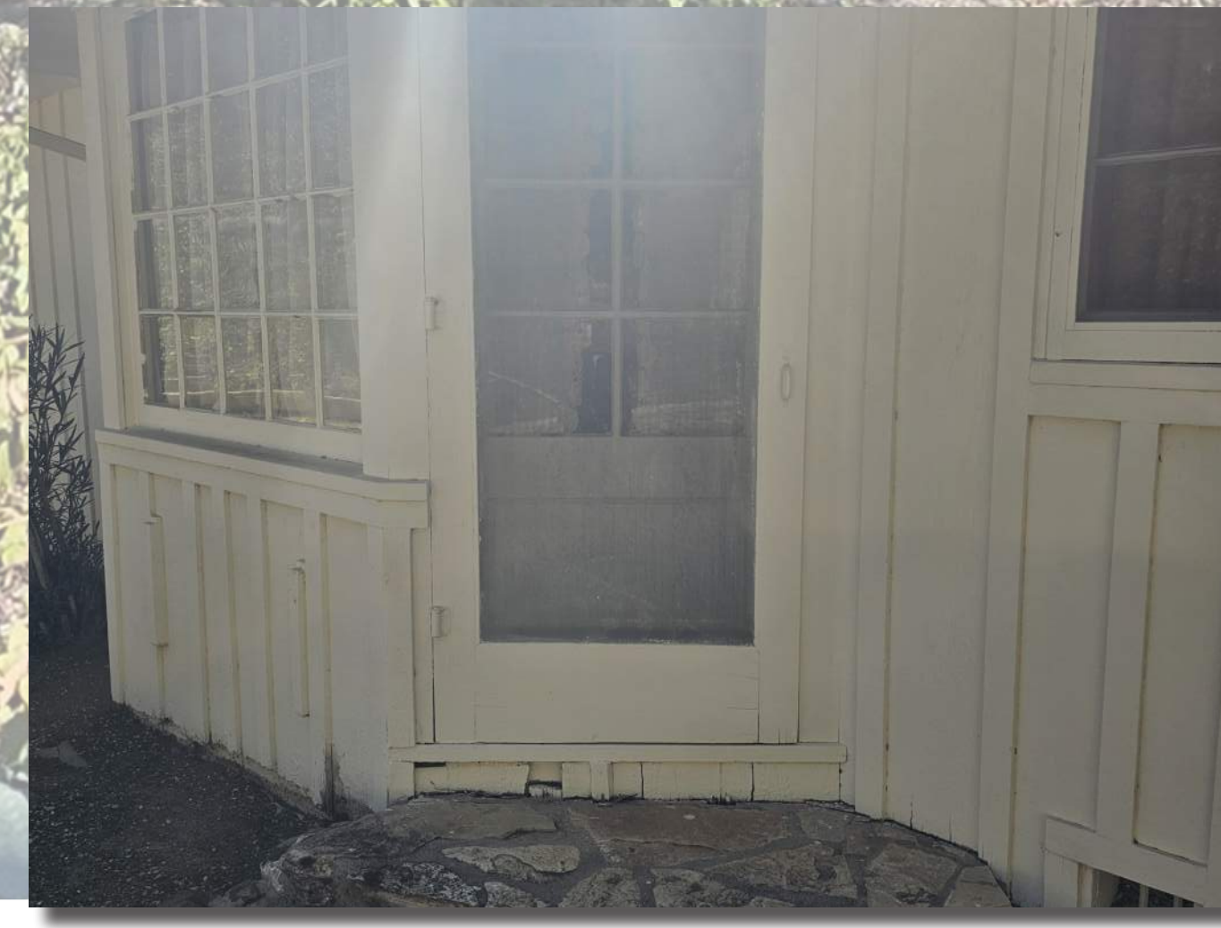
REPAIR/RESTORE ROTTED BOARDS ON EXTERIOR SIDING (2026 Est. Cost $12,000)
