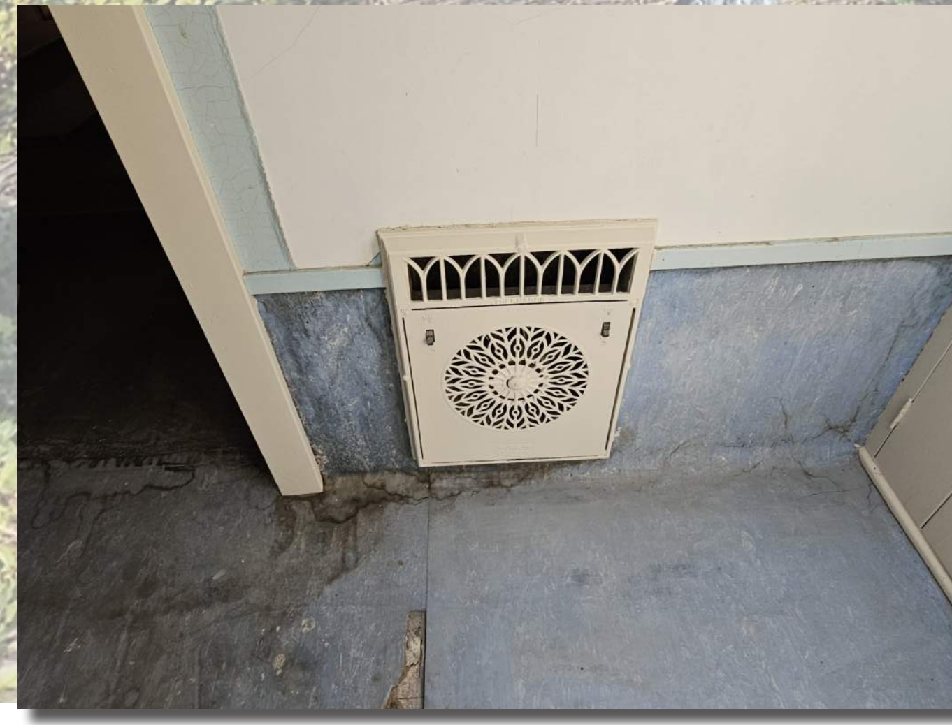
REPAIR/RESTORE HEATING UNITS (2026 Est. Cost $1,600)
