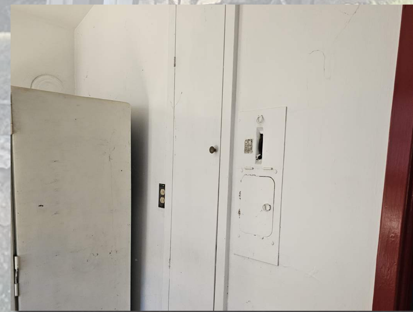
UPDATE ELECTRICAL THROUGHOUT HOUSE (2026 Est. Cost $1,500)
