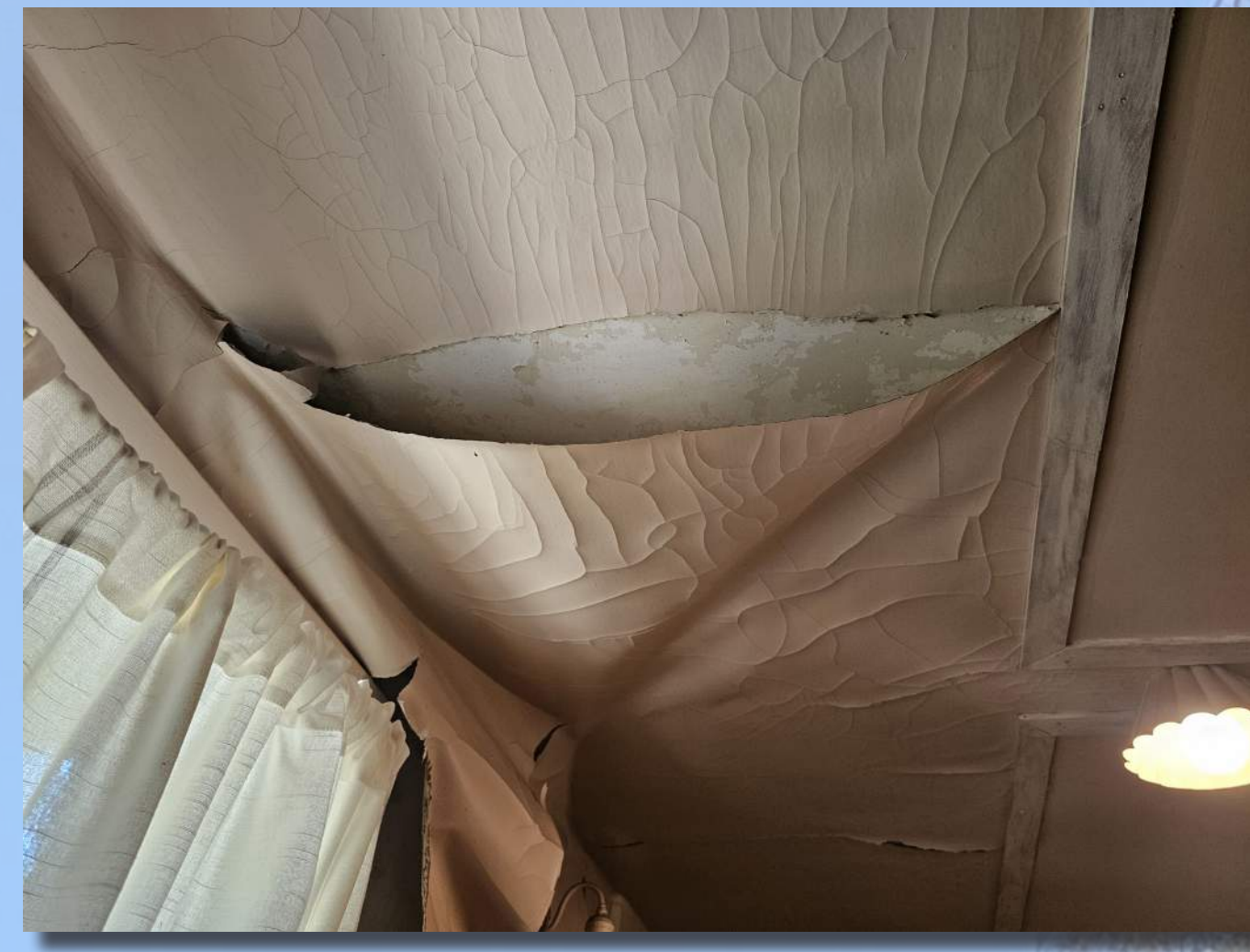
REPAIR/RESTORE WATER-DAMAGED CEILINGS (2026 Est. Cost $11,000)
