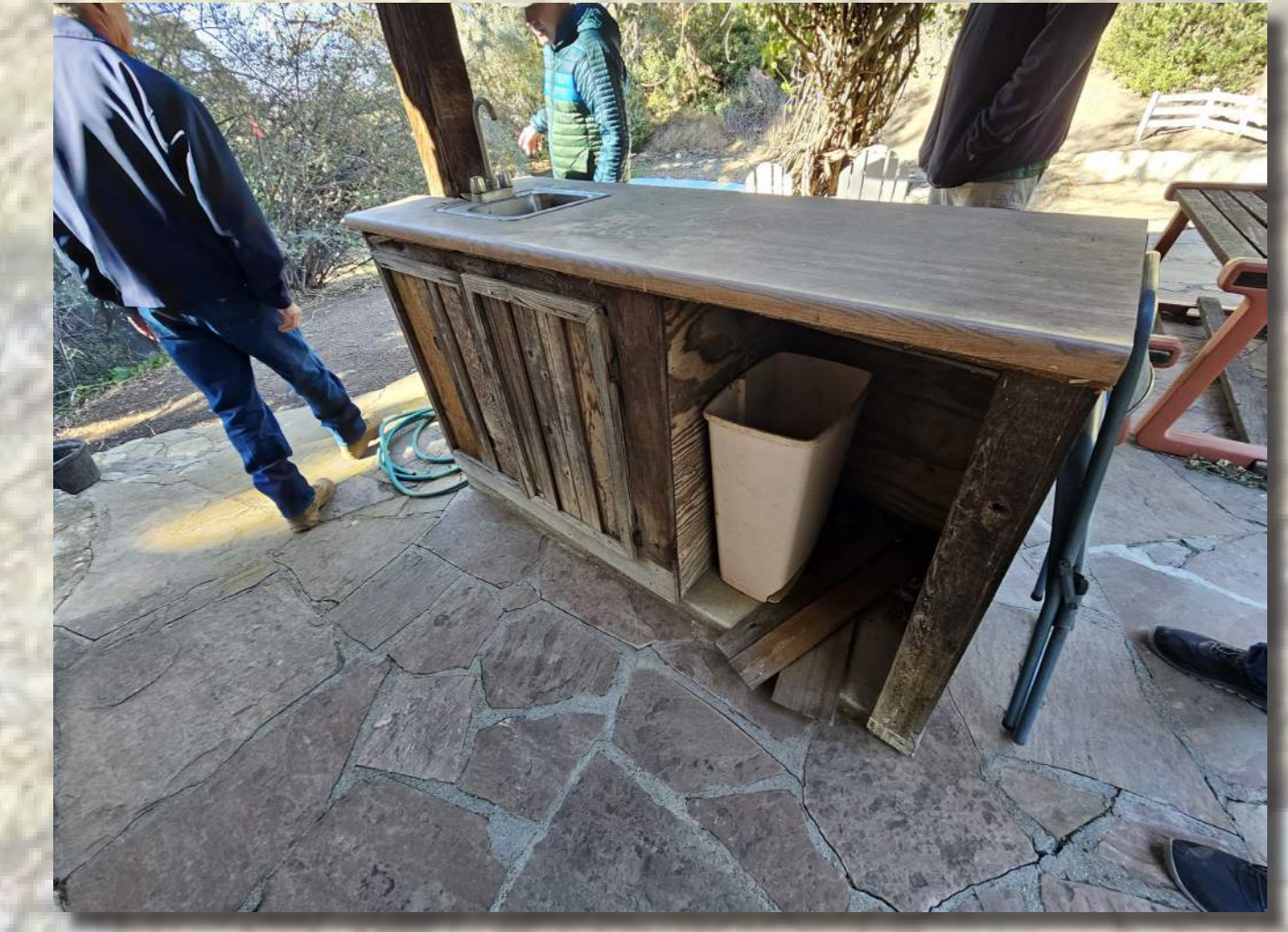
REPAIR/RESTORE FIXTURES AND EQUIPMENT (2026 Est. Cost $73,500)
